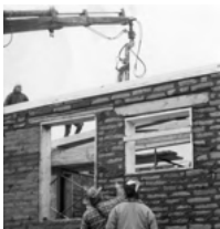
Constructing the Adobe House in M'Chigeeng, Manitoulin Island, n.d. Photograph by Carl Beam. Private collection. Courtesy of Anong Migwans Beam. © Estate of Carl and Ann Beam / CARCC Ottawa 2024.
