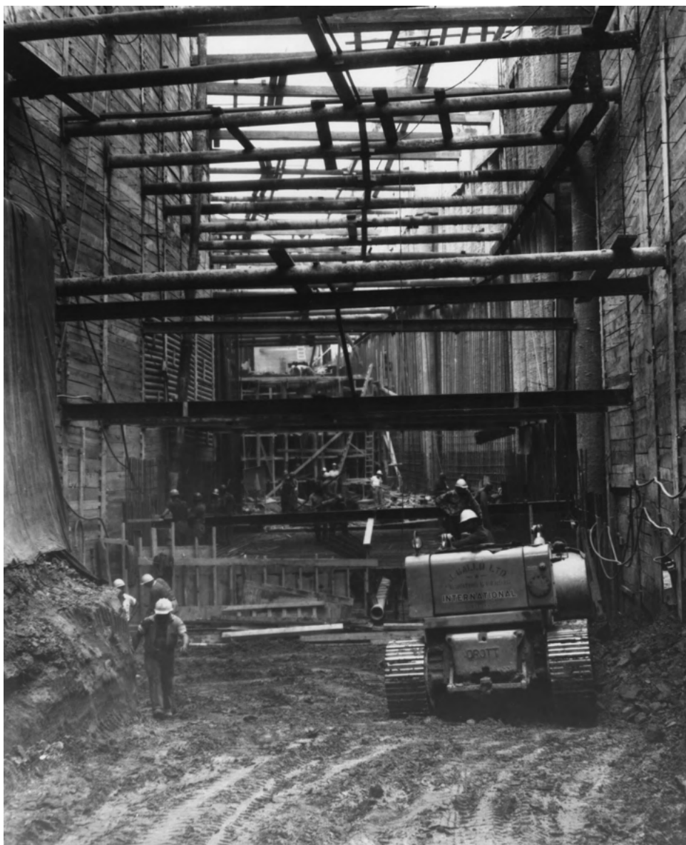
View looking south through the east leg of the wye connecting the University line with the Bloor-Danforth line, between Museum station and Bay station, June 27, 1963, photographer unknown, City of Toronto Archives.
